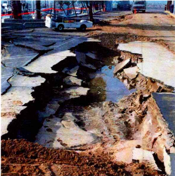
Liquefaction damage at Redondo Beach. Photo: CGS
